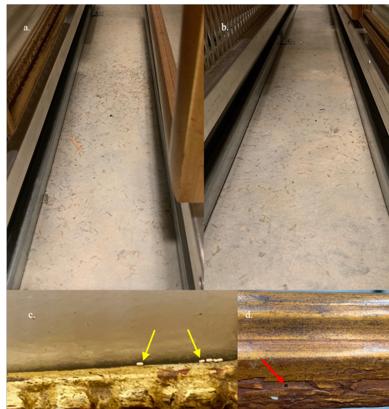
Figure 1. (a,b) Two rows of the vault floor showing the first sign of termite infestation—discarded termite wings. (c) yellow arrows—the drywood termite pellets, 1 mm in length, are shown on edge of the picture frame and (d) red arrow—the ‘knock-out’ hole, 1 mm in diameter, on the lower exterior portion of the frame.
